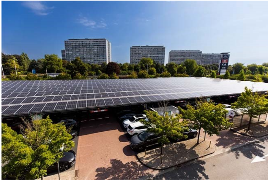
Figure 11: Carport with solar panels Waasland shopping center
